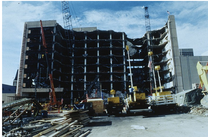
Figure 28. Partial collapse of Alfred P. Murrah Federal building [FEMA, 1995].
